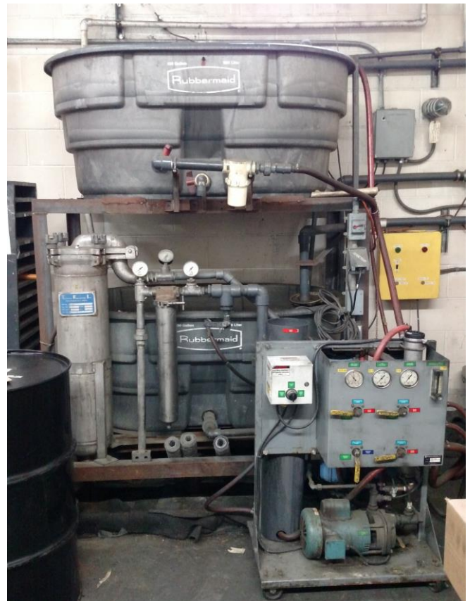
WRS System shown in foreground with two 150 gallon holding tanks in background; top tank for oily wastewater and bottom tank for clean effluent
